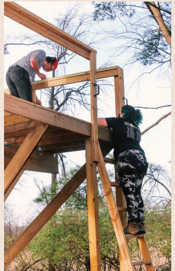
Owen and Seda work together to install the railing on the Tree Platform. Shaping Your Life members dreamed, designed and built the Tree Platform over the last 3 years for the community.
