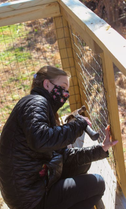
Shaping Your Life member, Caroline, works to affix wire netting to ensure the safety of the tree platform.
